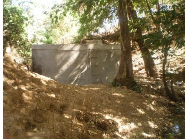
Fig: Storage reservoir
