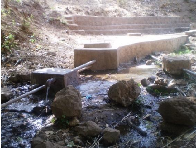
Fig: Spring box and outlets
