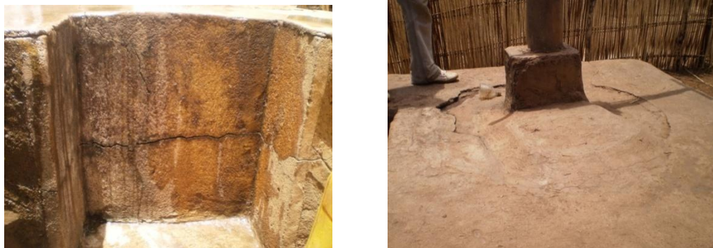
Figure 18: Cracks on head wall and top slab
