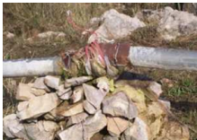
Broken systems, inadequate repairs
